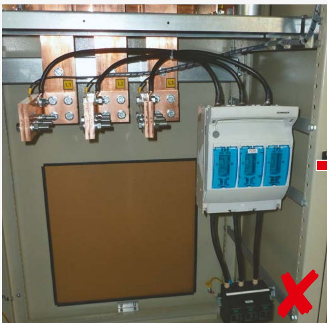
Before the intervention: The SPD installation fails to meet the condition as regards the length of supply conductors
