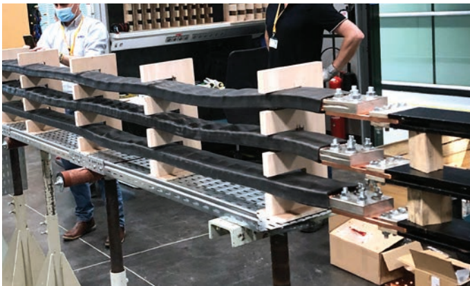
Temperature rise test sequence pictures and probe/temperature sensor all along the installation
